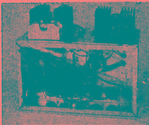
Fig. 10-27 — The heat sinks are mounted on an aluminum panel. When installing a power supply of this type, be sure to keep the heat sink fins in a vertical position to provide best air circulation. All of the filter capacitors are mounted in a row across the front of the chassis. RFC1 is located next to the transformer. Two sockets are mounted on the chassis side wall to accept an interconnecting cable from the transceiver. To the left of these sockets is the bias voltage adjustment control, R3. This model of the power supply was built by W8HS and assistance was given by W8DDO, W9IWJ (of Delco Radio Corp.), and Jim Osborne (of Osborne Transformer Co.).
